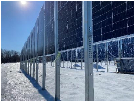
Sunzaun's racking system installed at the Rutgers Animal Farm.
